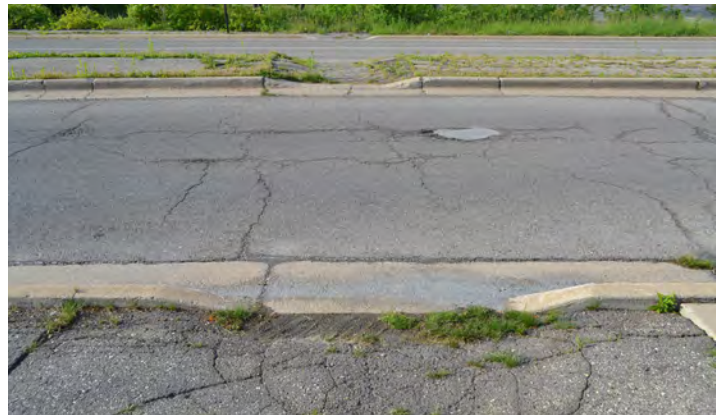
Sidewalks and pedestrian crosswalks are deteriorated
